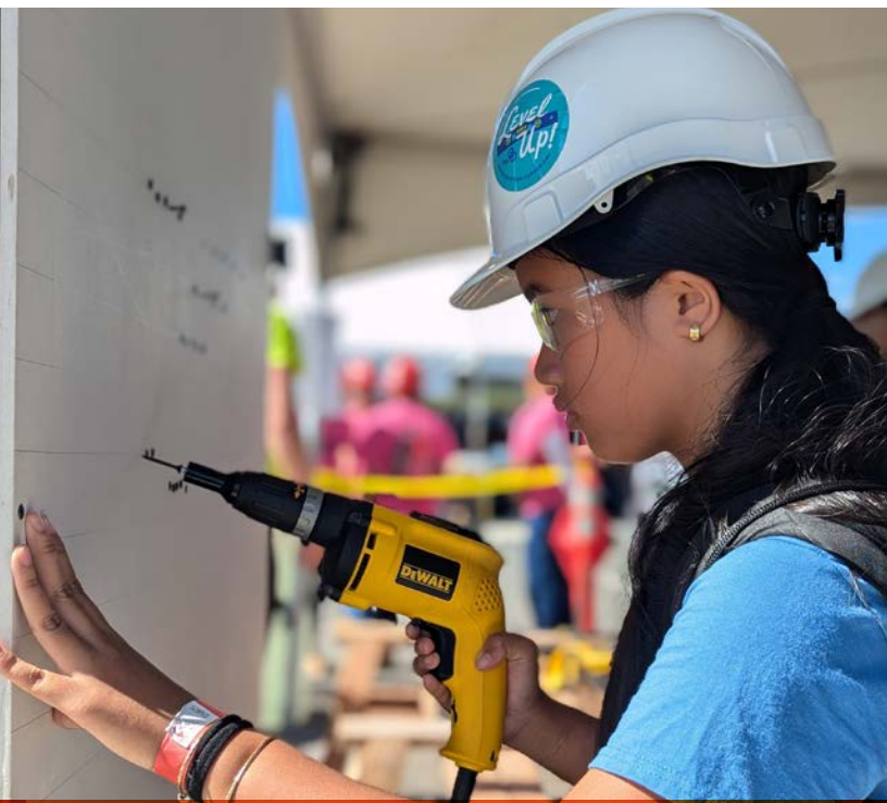
Precision Learning: A high school student practices drilling screws into drywall, gaining hands-on experience with essential construction skills.
