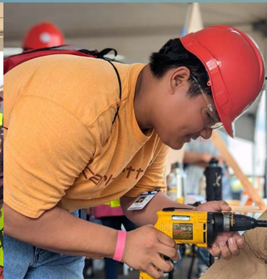
Focused & Determined: Students tried their hand at HCATF's drywall station to learn trade skills.
