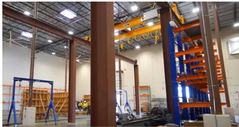
2090 houses specialized equipment, where apprentices can hone their skills through hands-on training.
