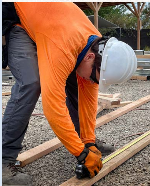
Summer intern Mitchell Naeole Jr measuring at the prefab yard with Gill Construction
