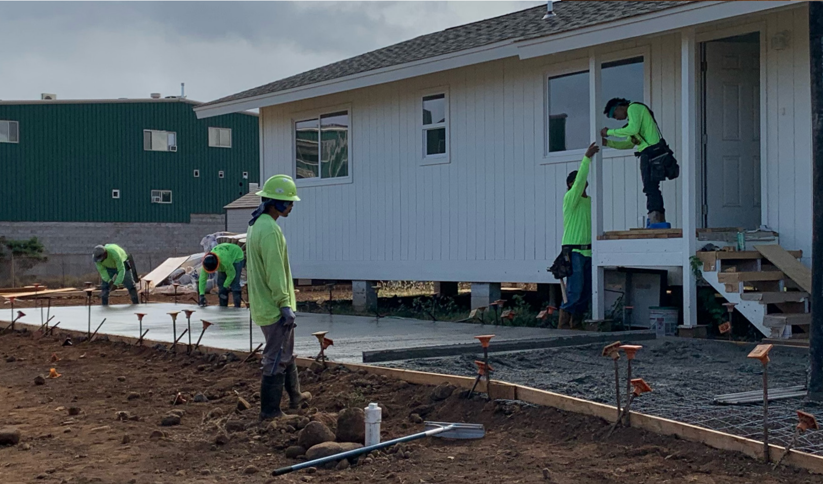
HCATF's Rough Framing class constructs front door handrails, while the Concrete Form class installs slab-on-grade formworks.
