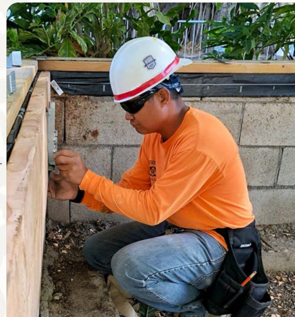
DEDICATION TO DETAIL: An apprentice installs joist hangers in the beginning phases of the project.
