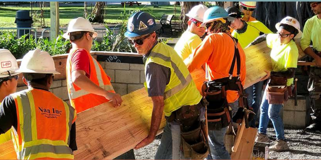
TEAMWORK MAKES THE DREAMWORK: Rough Carpentry instructor George Boeman and his students worked together to accomplish some heavy lifting replacing the glulam beam for the stage.
